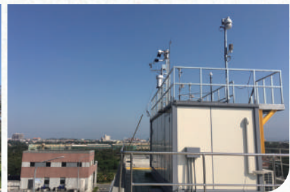
Longtan Science Park-Longtan Service Center Station
